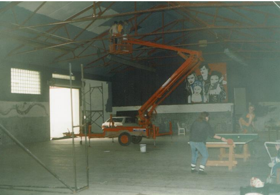
Time for a quick game of table tennis while work continues above.
